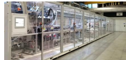
Westchester Facility Filling Machines
