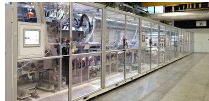
Westchester Facility Filling Machines
