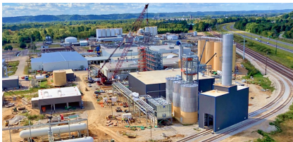
Ironton Production Plant
